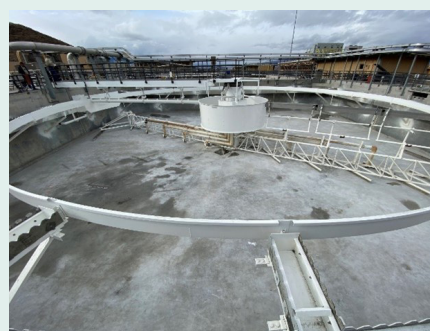
Clarifier ready for recommissioning with a fresh coat of paint on all steel components and a new layer of concrete grout on the tank floor.
