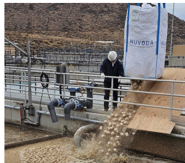
Kenaf media being added to the Activated Sludge process at TMWRF. Staff added thirty-two (32) bags weighing 1,500 pounds each over the course of two days.
