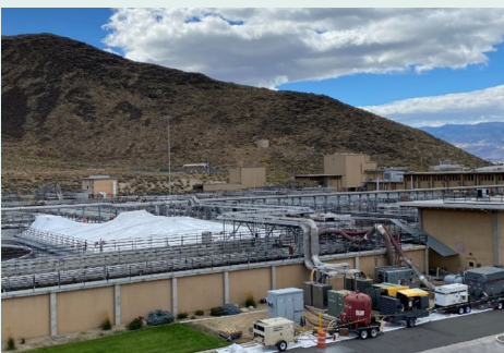
Containment tarp built around the clarifier complete with dust collection and humidifier. The steel inside the tank is blasted with a sand-like media and recoated. This containment keeps everything inside the job-site while the auxiliary equipment keeps the conditions safe for work under the containment.
