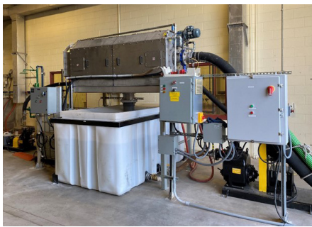
Equipment installation for MOB demonstration at TMWRF.
